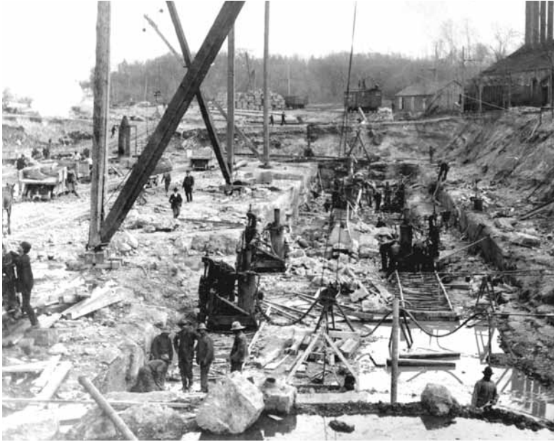
Canadian Niagara Power Plant workers excavating through rock for the wheel pit, 1902. Courtesy of the Niagara Falls (Ontario) Public Library (D415450C).
